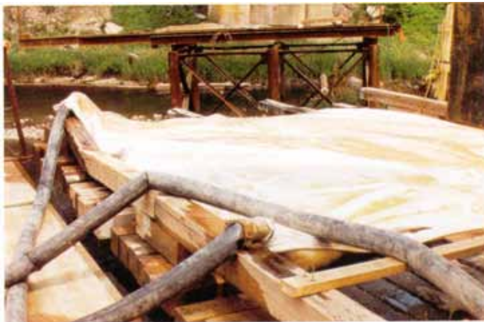
Filter bag installed on temporary access structure before start of dewatering operation
