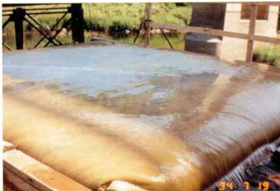
Filter bag after start-up of dewatering operation. The sediment is retained in the bag and the bag is disposed of at an approved disposal site after use.
