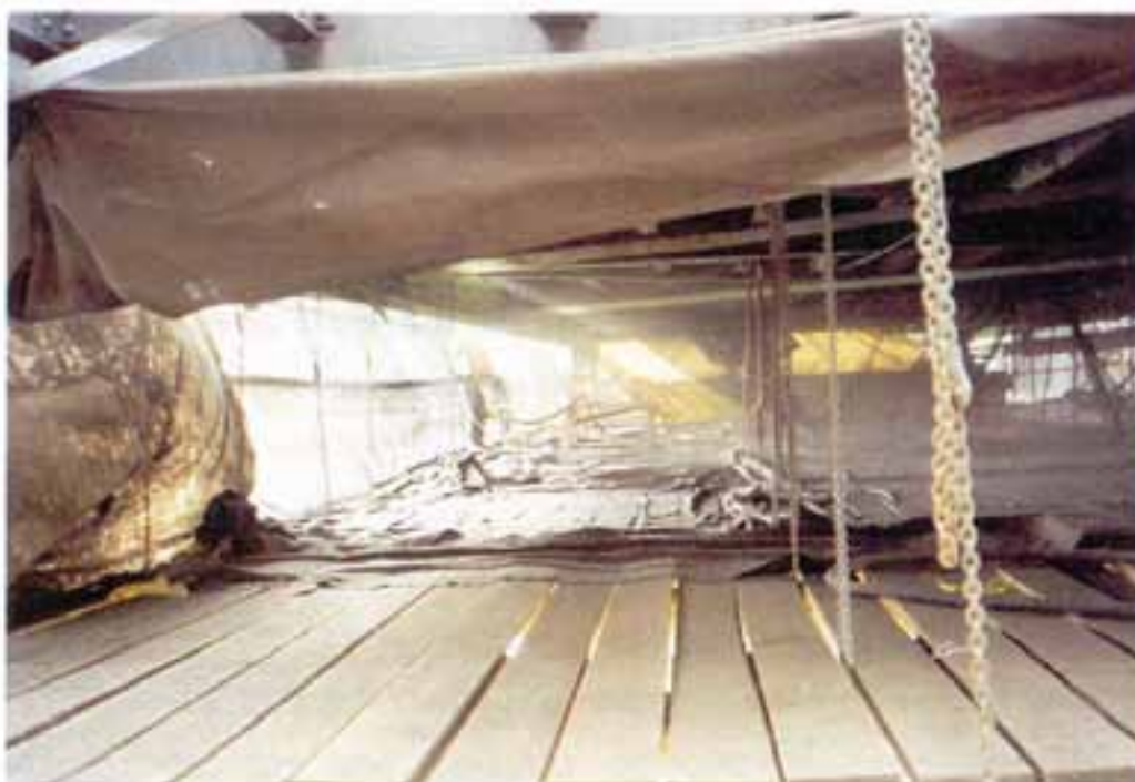
Typical set-up for below deck work. Note geotechnical fabric over staging to allow for collection of spent abrasives.
