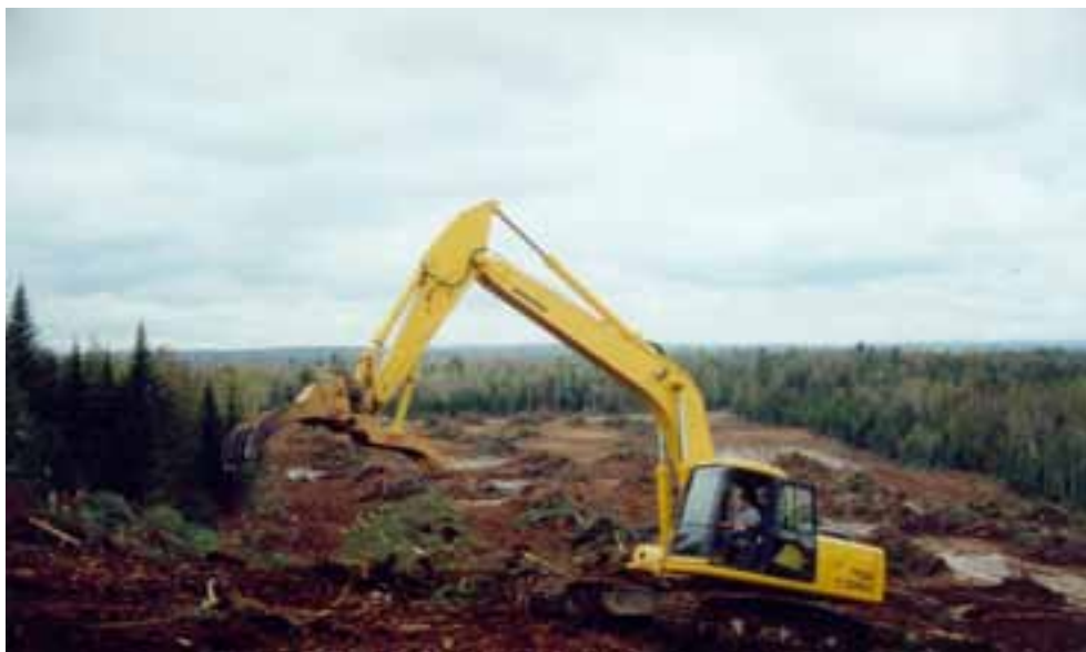
Root rake attached to excavator used to remove roots and stumps only.
