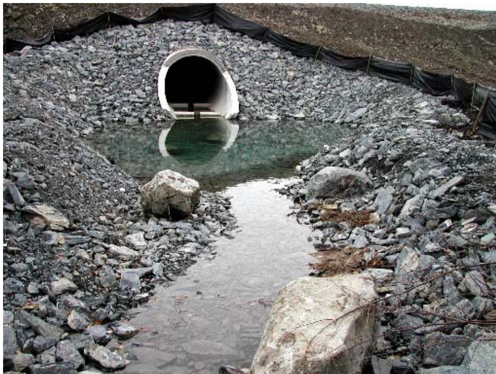
Riprap used as culvert protection and channel protection.
