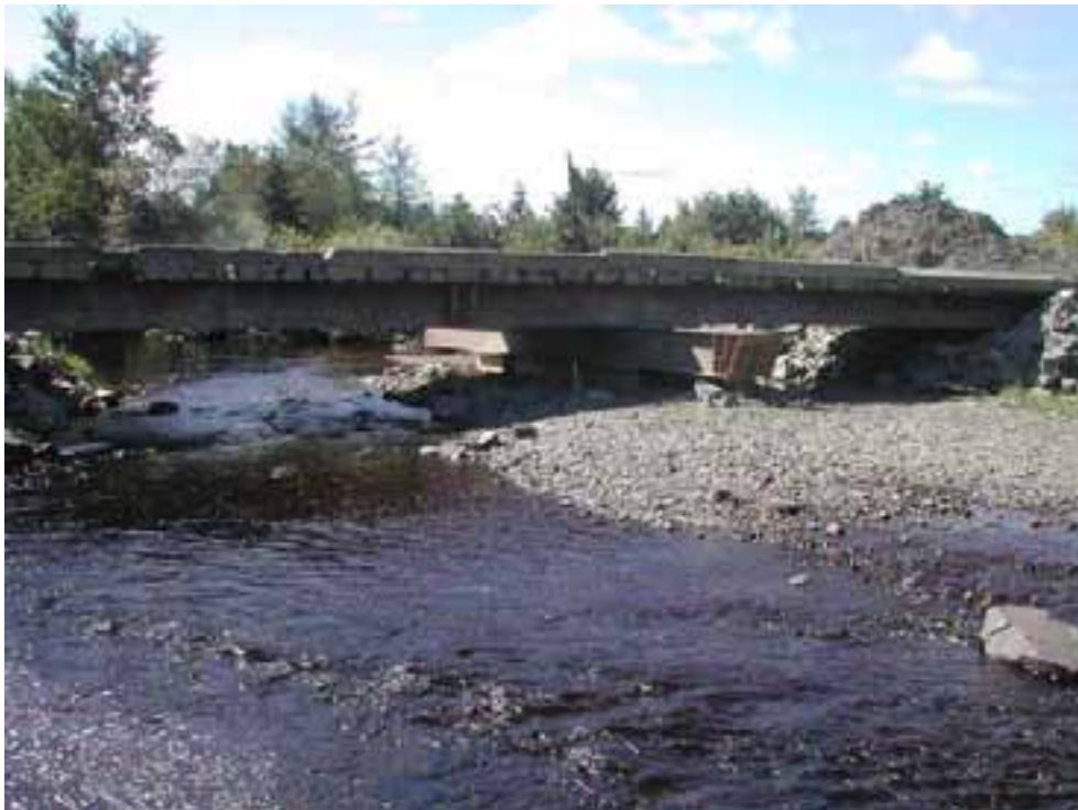
Temporary crossing at narrow location. Note sideboards on structure to limit the amount of debris that can enter the watercourse.
