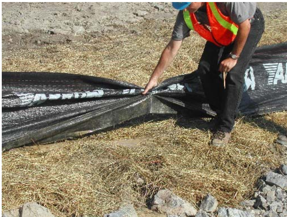
Sediment control fence not properly installed
