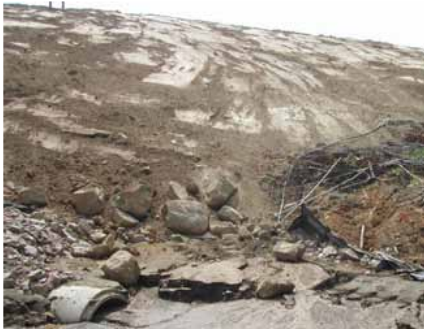
Large rocks have buried the fence allowing sediment to pass over.
