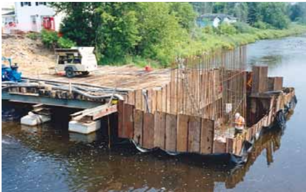
Sheet-pile cofferdam and filter screen at bridge pier location to isolate the work area from the watercourse.
