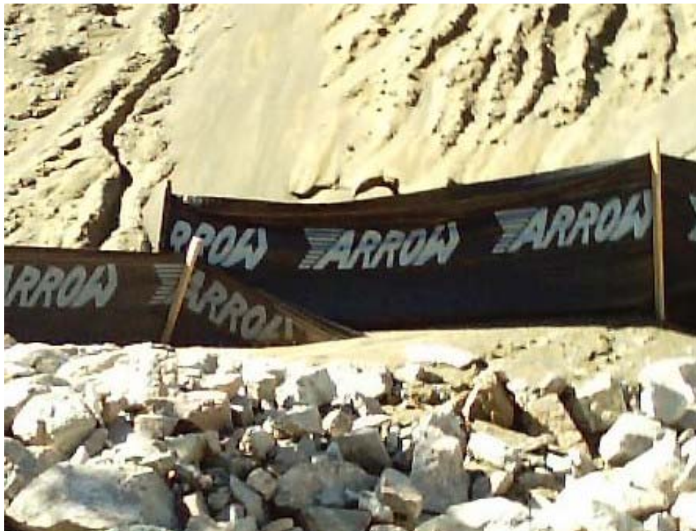
Sediment passing around end of fence.
