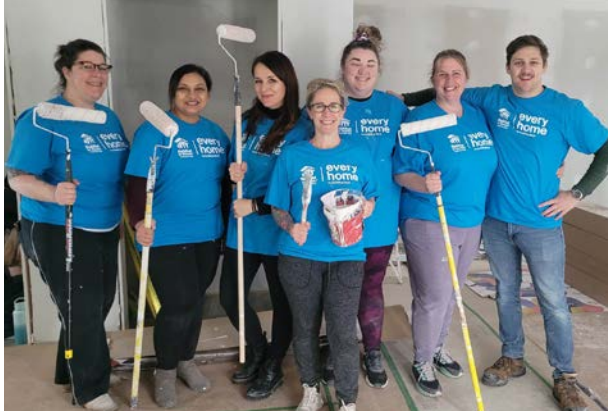
Volunteers for Habitat for Humanity Fredericton Area lend a hand to paint two duplexes on Devon Avenue and Titus Street. The recycled paint for both homes was generously donated by Laurentide Re/Sources.
