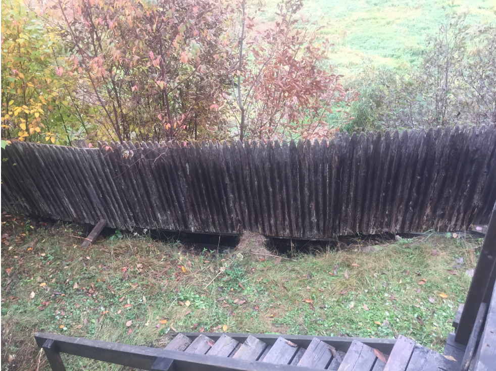
Figure 4: Two Photos of Erosion at Base of Fence. Retaining Wall on Opposite Side.
