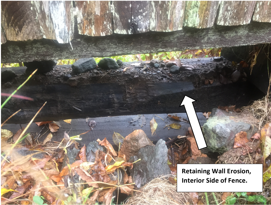
Figure 5: Existing Retaining Wall at Base of Fence Damaged by Spring 2018 Flood
