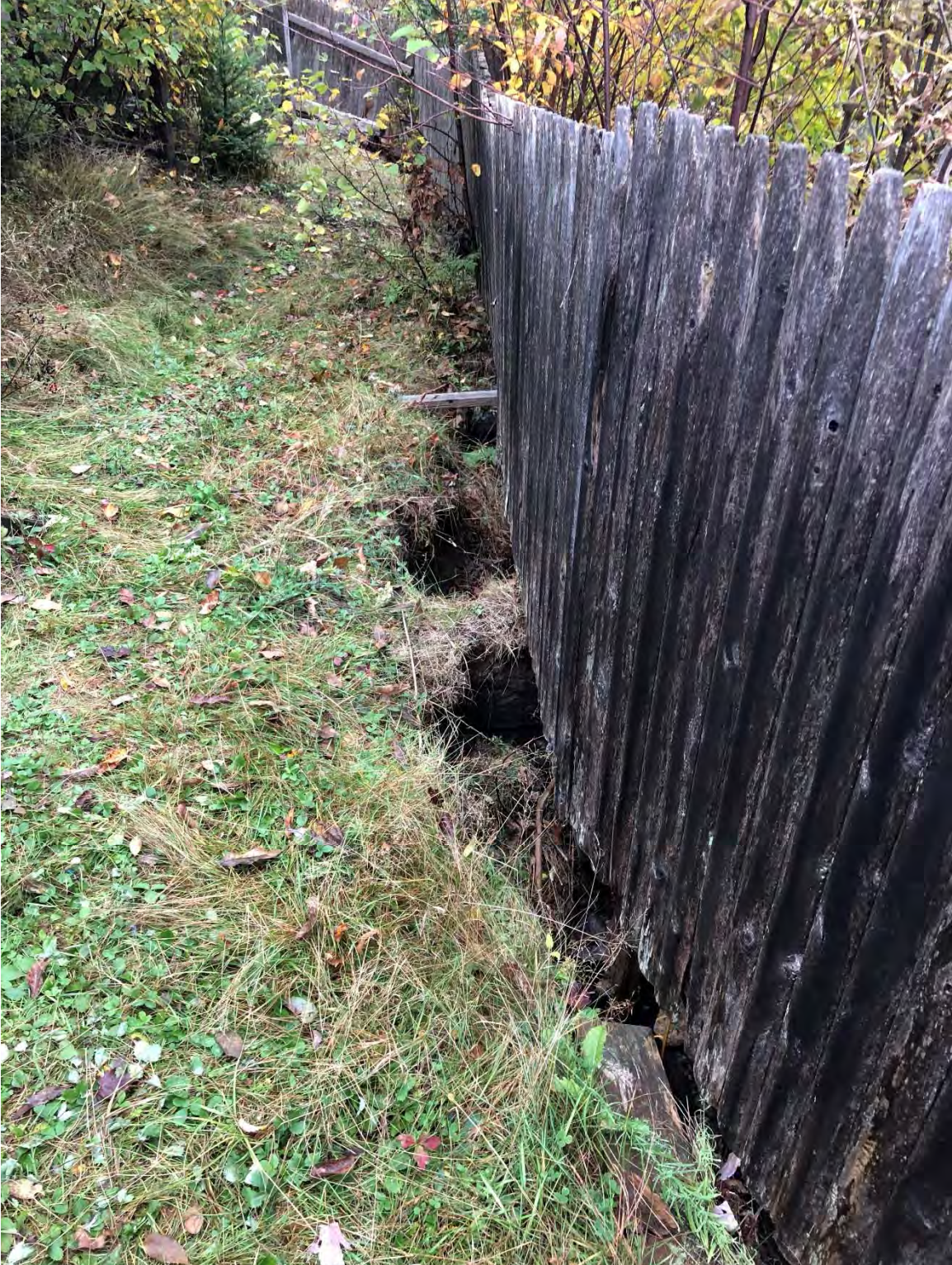
Figure 14. Photograph taken on 12 October 2018 looking along the fence at the edge of the cribwork retaining wall at 11 Southers Road in Bayswater, New Brunswick.
