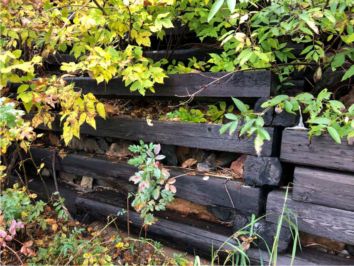
Figure 13. Photograph taken on 12 October 2018 looking at a portion of the cribwork retaining wall at 11 Southers Road in Bayswater, New Brunswick.
