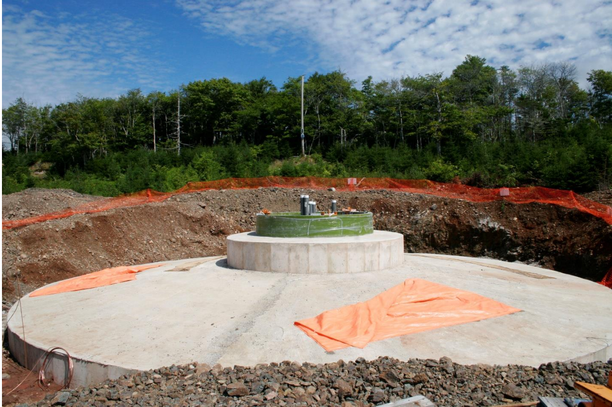
Figure 2-4: Finished concrete foundation for Natural Forces' Fairmont Wind Farm in Nova Scotia
