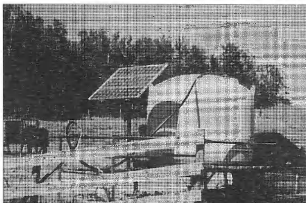
Solar powered pump in use.
