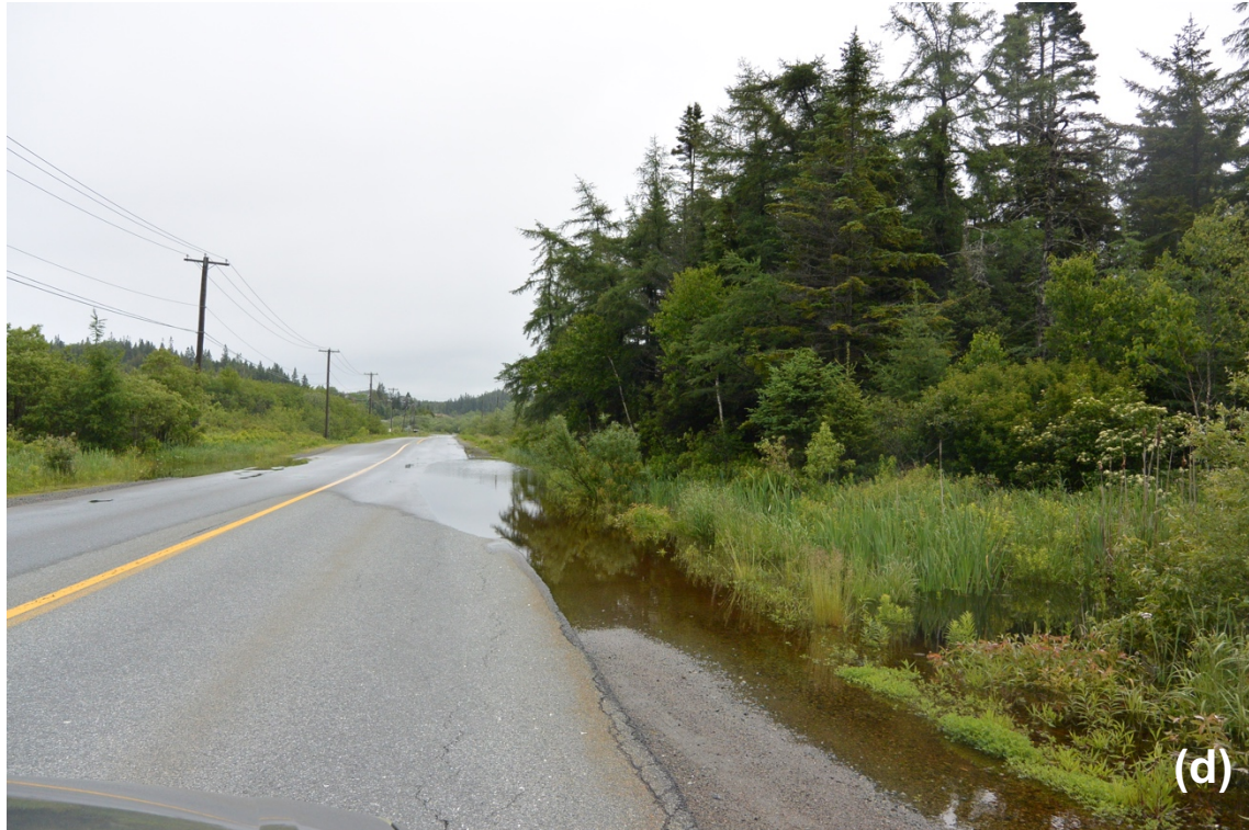
Figure 5. Aftermath of a major rainfall event on June 28, 2018 (65.5mm of rain) in Little Marsh Creek within the proposed project area. (a) Flooding near the culvert (45.32282, -66.03483). (b) Flooding along the stream near Ashburn Road (c&d) Flooding on Ashburn Road.
