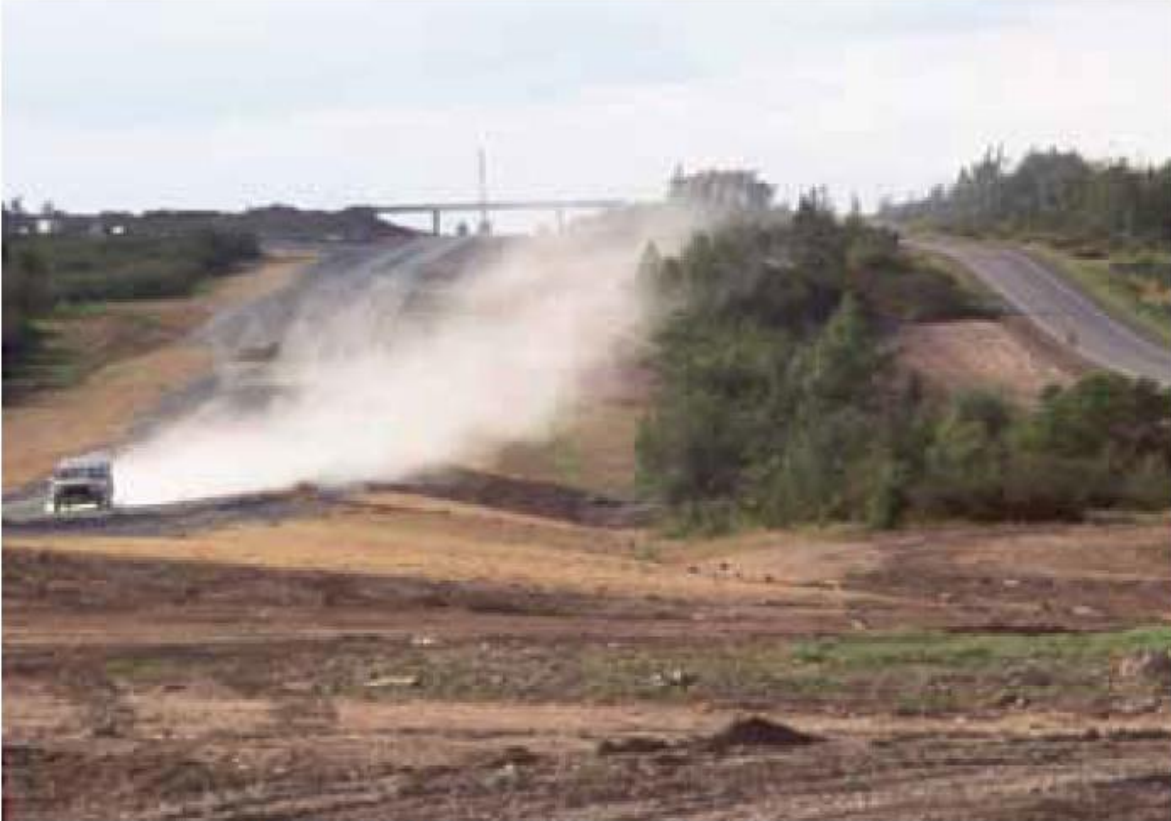
Worksite that requires dust suppressants.
