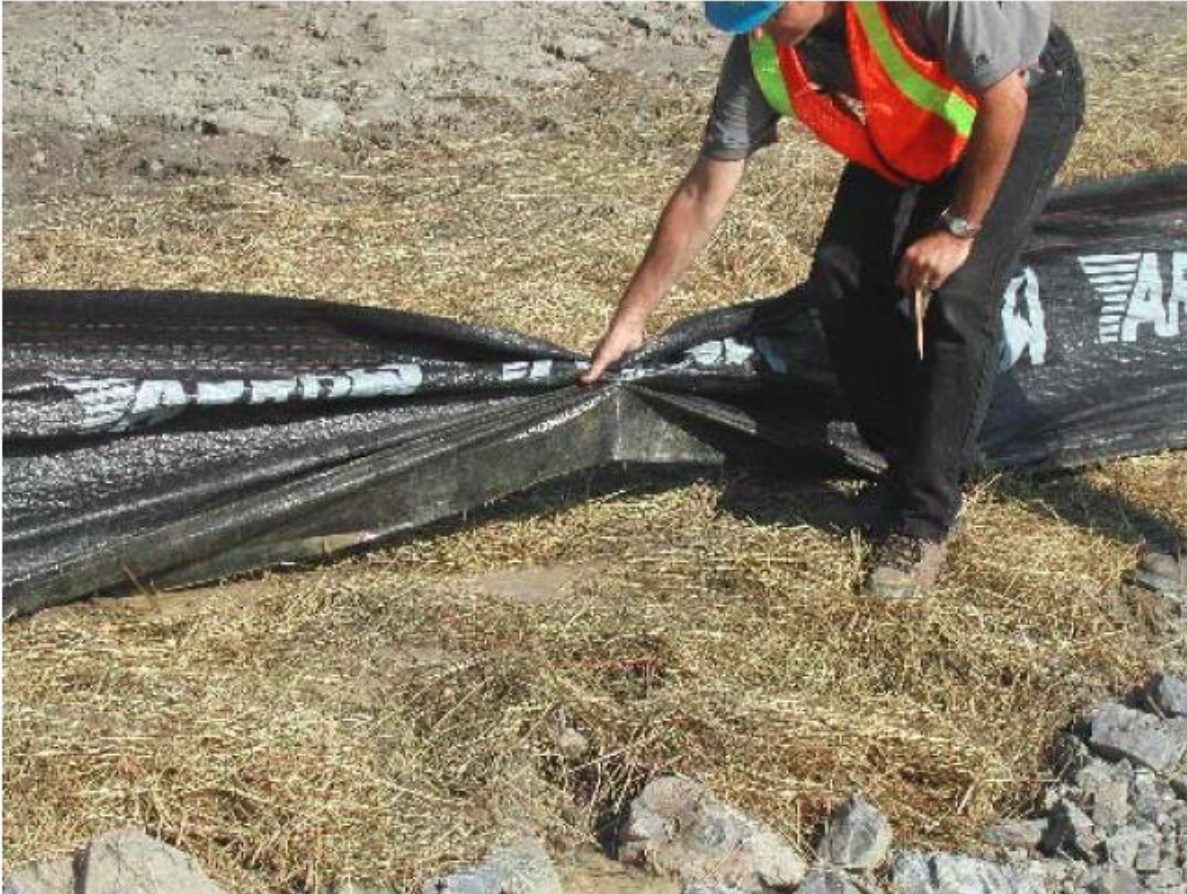
Sediment control fence not properly installed
