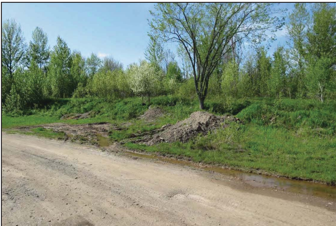
PLATE 7: Fill stockpile covering the proposed site of the water treatment facility; facing northwest; May 29, 2014.
