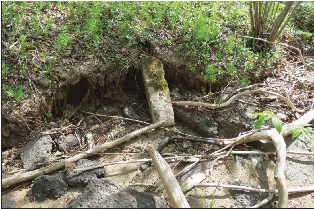
PLATE 4: Eroded bank along Saint John River. Note chunks of asphalt and concrete from nearby refuse deposits; facing south; May 29, 2014.
